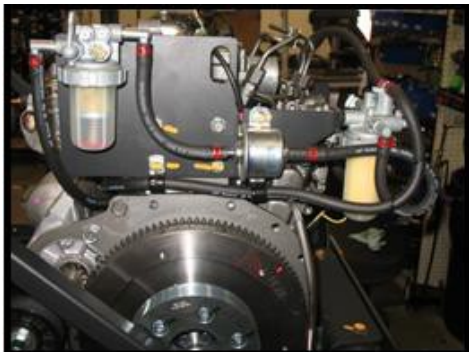
Filters and Fuel pump (Installed)
